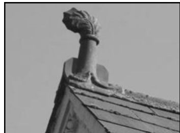
Original finial - smoke emerging from chimney?
