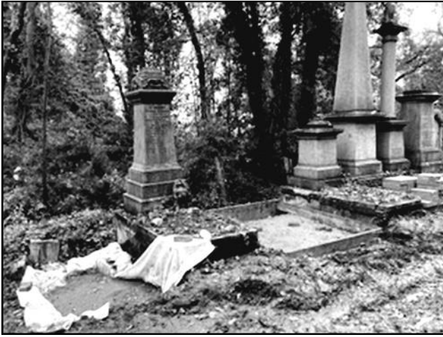
Memorials under repair on Dissenters Road. Here the vaults have been in-filled with shingle and new concrete pads installed on which the original memorial will be placed. Note the mud!
