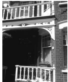
Fig 6. A porch on Mulgrave Road, Dollis Hill Estate, with original trellising and balustrade
